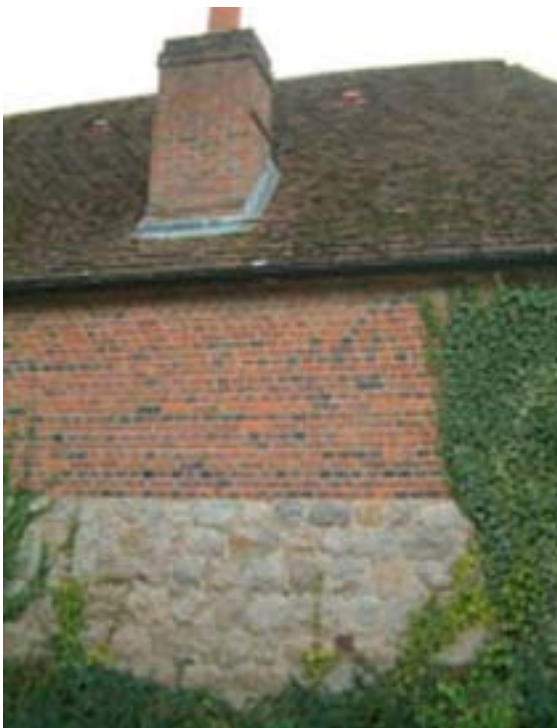
A sarsen stone farm building raised in the early 19 th century to 2-storeys with chequered brick and a chimney added for a dwelling.
