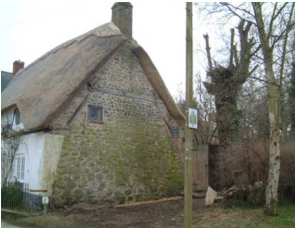
Timber cruck frame in a sarsen stone gable wall and in the foreground the historic village pound
